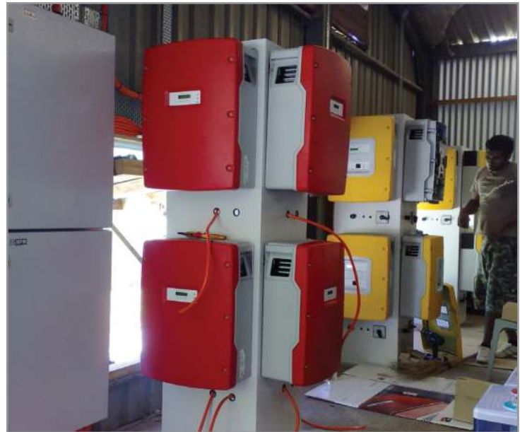
Figure 6: Battery banks and inverters.
