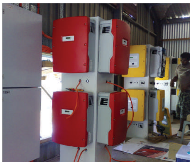
Figure 6: Battery banks and inverters.
