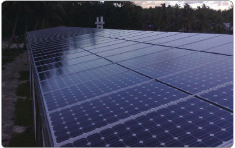
Figure 5: Solar panels on grandstand roof at the Motufoua School Stadium
