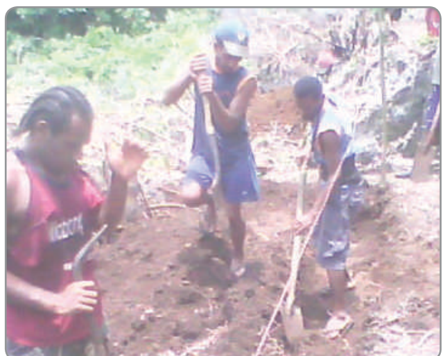
Figure 11: Digging the trench for the Talise hydropower system (Photo taken in November 2011)
