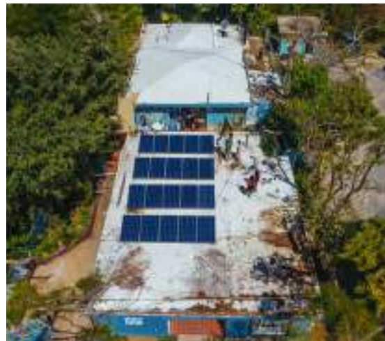
Solar panels, Community center.
