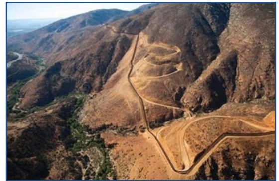
Photo: Mt Olay A draft environmental impact statement (EIS) prepared prior to wall construction stated that constructing a wall in this area would have long-term impacts on its flora, fauna, and water resources. The EIS warned that grading and road construction associated with the wall (prohibited in wilderness areas) would remove layers of topsoil and destroy fragile, intertwined plant roots that protect chaparral habitats from
