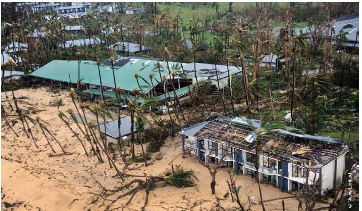
Damage and mass sand deposition at Dunk Island Resort caused by several metre storm surge during TC Yasi.
