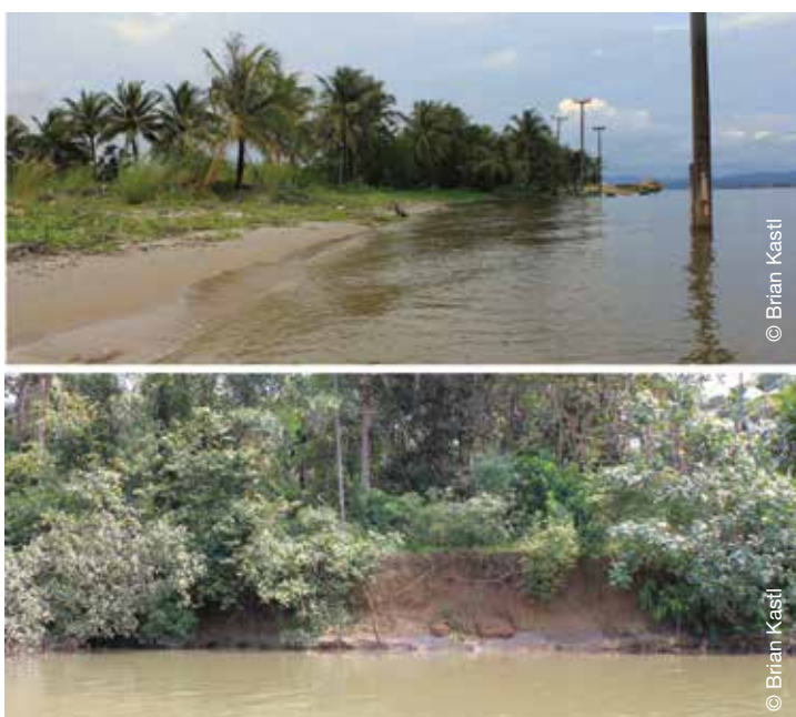
Figure 12: Estuary erosion (top) left power lines in the water 2 km west of Koh Kong city. River bank collapses 1 km north of PKWS in the sand mining region (bottom).
