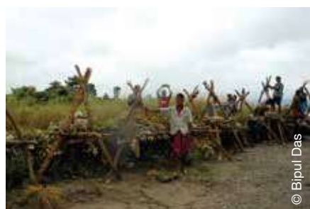
Step 4: Construction of deflectors (called porcupines) using locally available materials and through collective labour.
