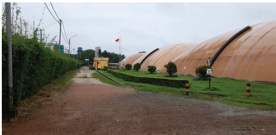
Methane capture facilities for palm oil mill effluent for electricity generation, Belitung, Indonesia Photo: Erik Meijaard
