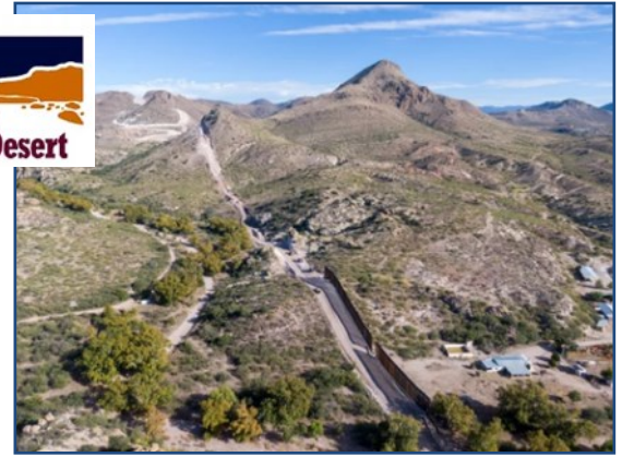
A portion of the border wall under construction in Arizona's Guadalupe Canyon, a wildlife corridor for Mexican gray wolves & endangered jaguars. USA on left. John Kurc NPR Nov 2020
