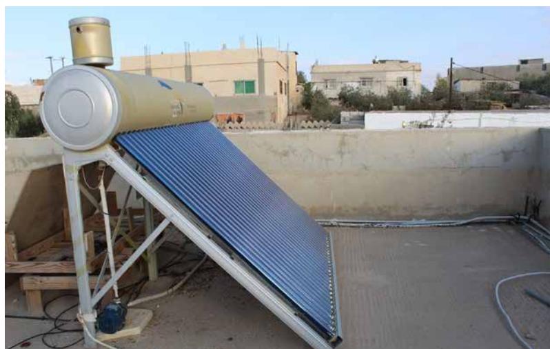
installed solar water heaters / cc: IUCN ROWA
