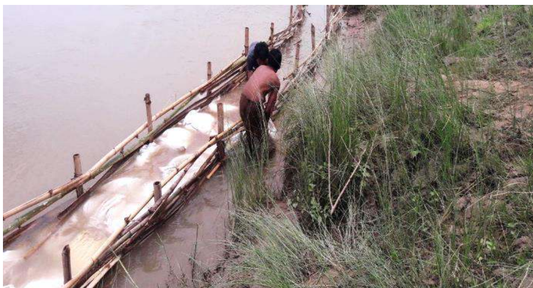
Figure 26: Riverbank stabilisation activities applying bamboos and grass plantation in Chaudhar River, Nepal ©Kishan Khadka
