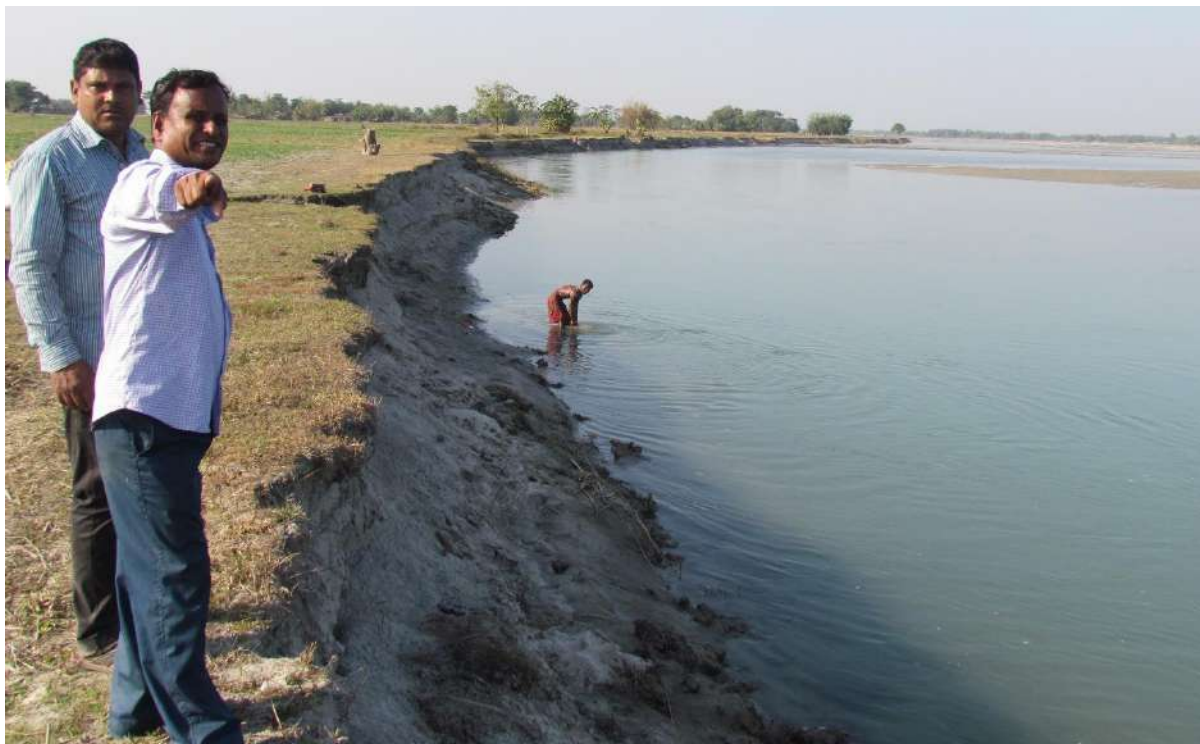
Figure 22: Local villagers sharing the problem related to river bank erosion in Padamati Char, Teesta River, India ©MAUSAM
