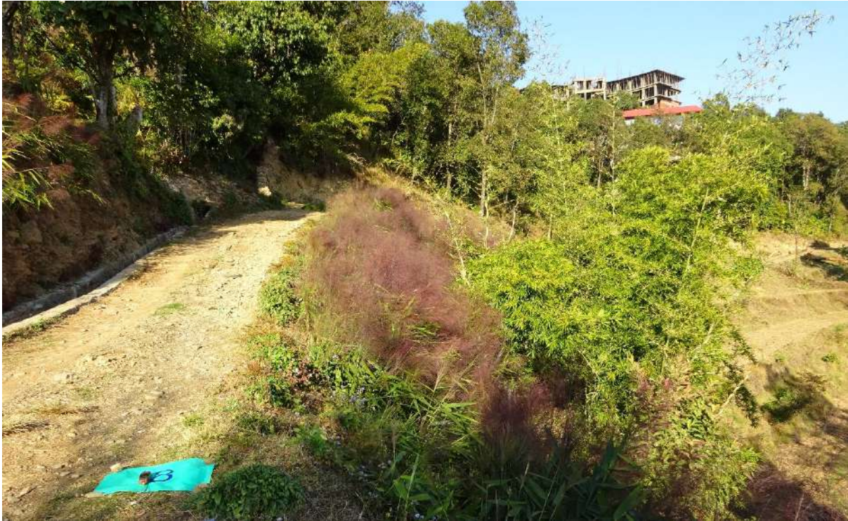
Figure 21: Eco-safe roads after two years of project intervention with lush green grass growth along the sides ©ESR Nepal
