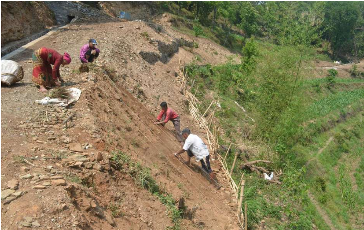
Figure 19: Villagers preparing site for the demonstration of eco-safe roads in Gharelu Village, Nepal ©Sanjaya Devkota
