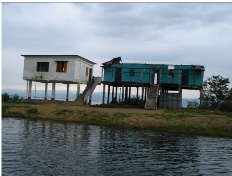
Left: New rest house constructed by LGED upon request from THMC Right: Old rest house recently damaged by cyclone requires repair
