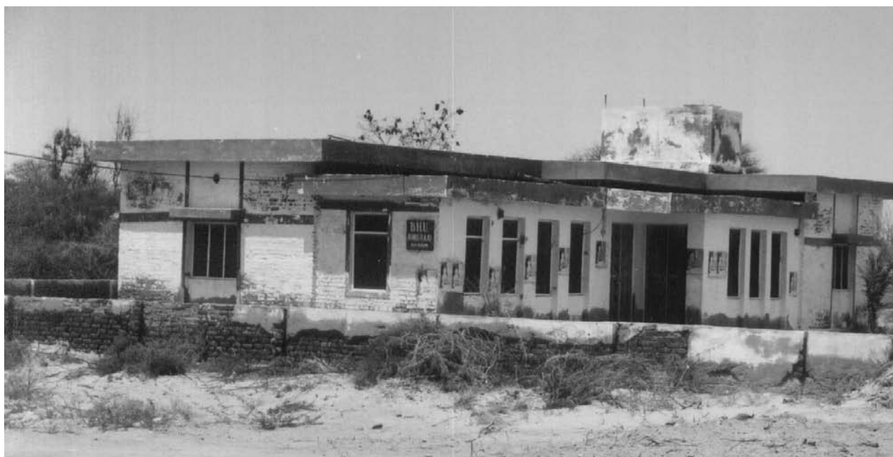
A dilapidated BHU at Ahmed Rajo.
