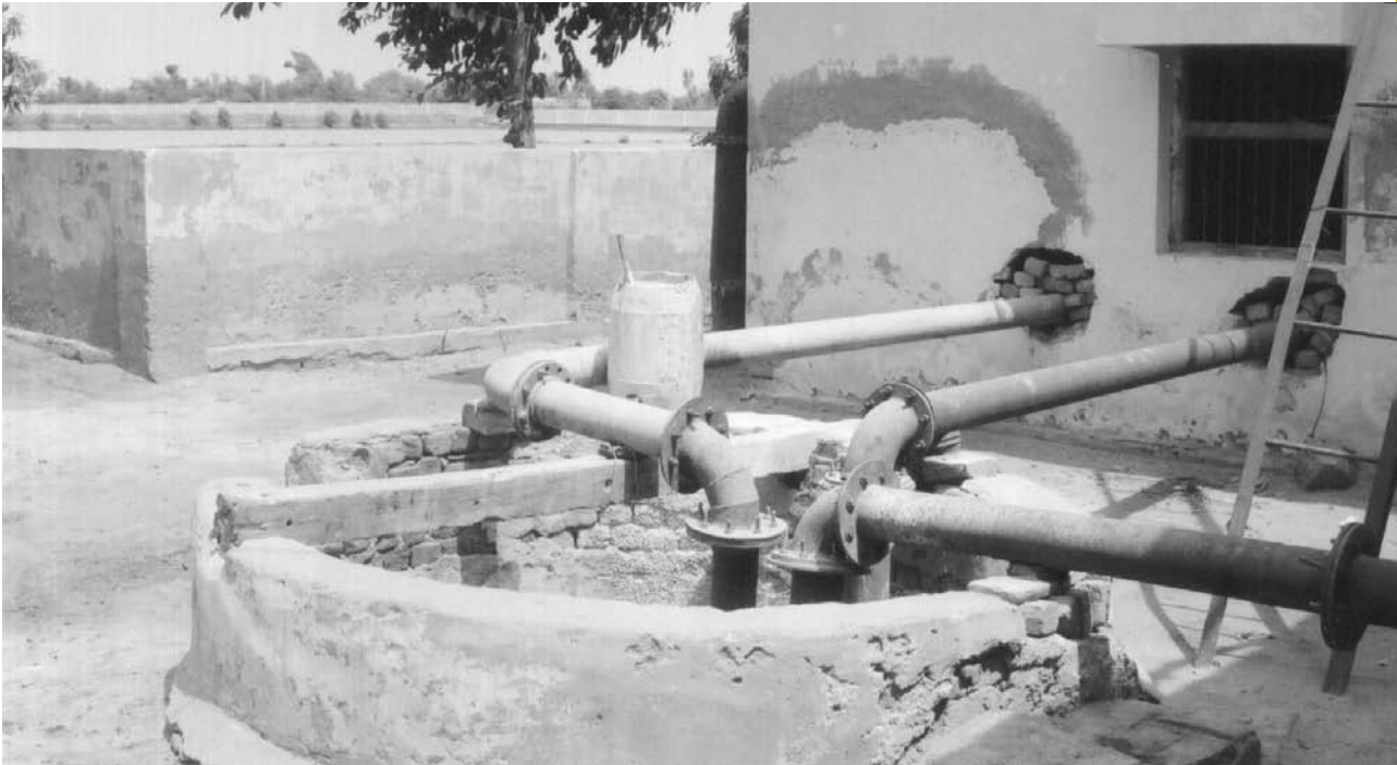
Provision of drinking water needs immediate attention.
