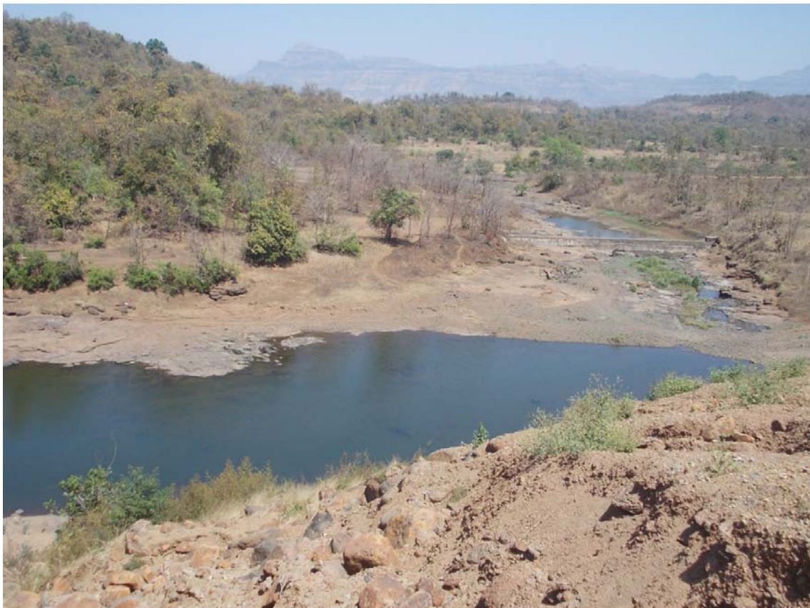
Figure 13 The site of construction for the Kalu drinking water project on river Kalu, near Thane district, Maharashtra (Shiba Desor)
