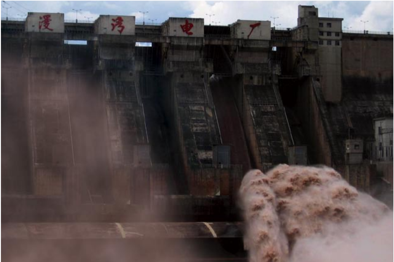
Manwan Dam, the first hydropower project on the Lancang-Mekong River in China. © IUCN
