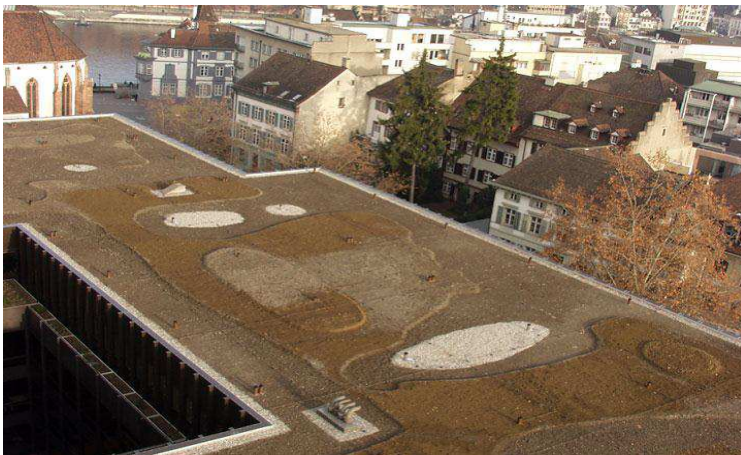
Newly constructed green roof on the Klinikum 2 of the Cantonal Hospital of Basel, built in accordance with the city's new guidelines on green roofs and urban biodiversity – (Photo Brenneisen) http://www.ieep.eu/assets/903/GI_Case_Analysis_5 - Urban Green Infrastructure.pdf
