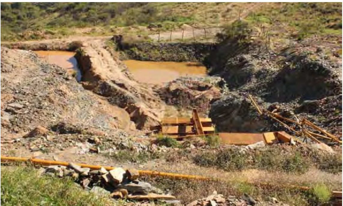
First gold mining site within JML's ML. Closure work has yet to start (photo 4.16).
