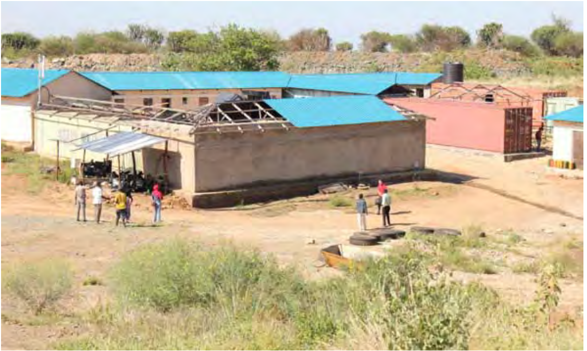
Jan Mangal's office at Nakabat Gold Mine, showing roofs necessitating repairs. Surrounding areas show extensive vegetation clearance, bare soils and presence of pioneer/exotic plant species (photo 4.10).
