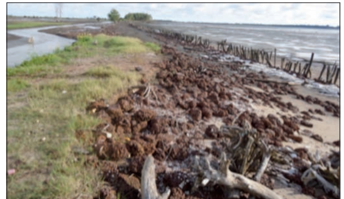
View of a clogged sea wall
